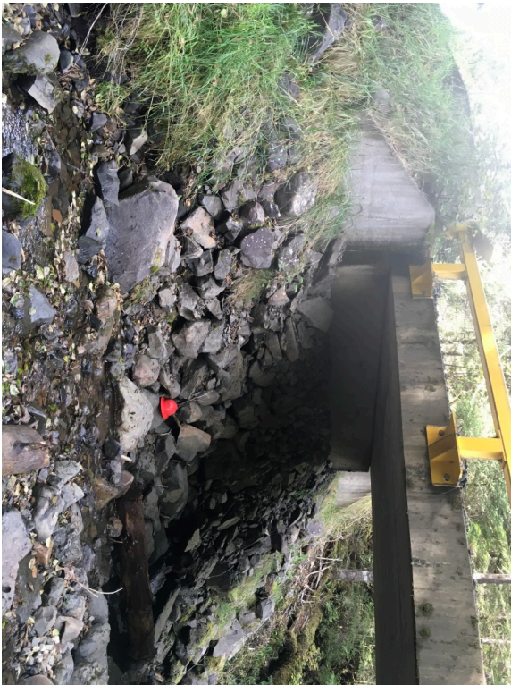
Scoured riprap on left bank
