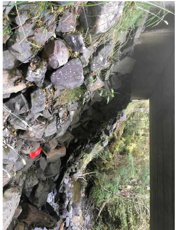
Scoured riprap on left bank
